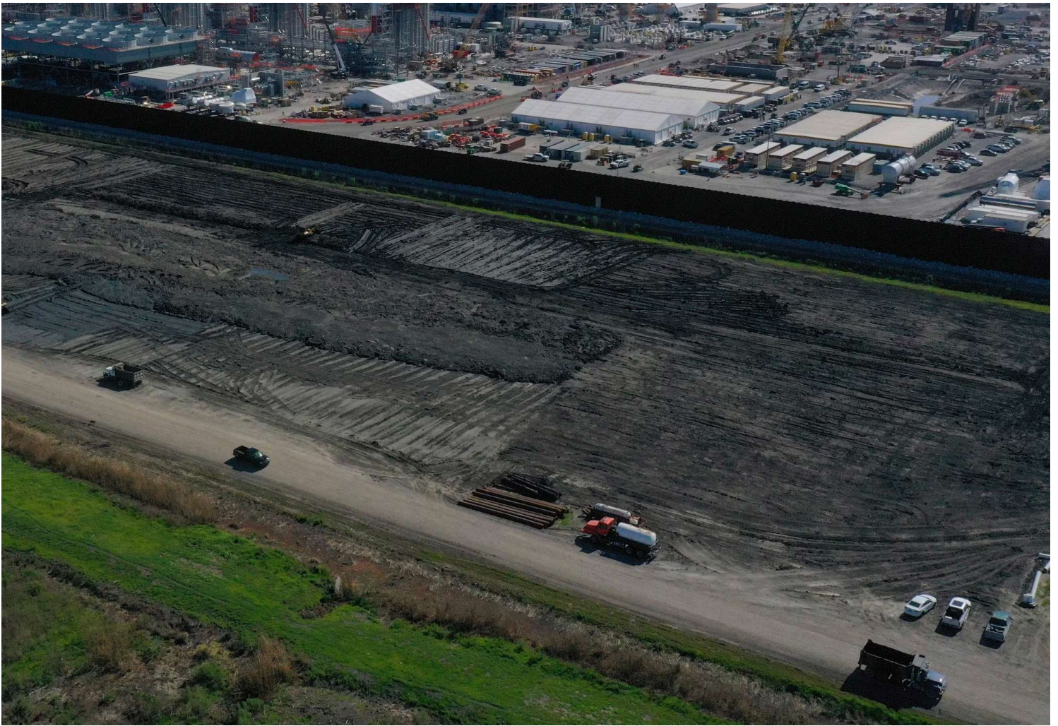
An aerial view of the ongoing construction at the Plaquemines LNG export facility in Port Sulphur, La.
